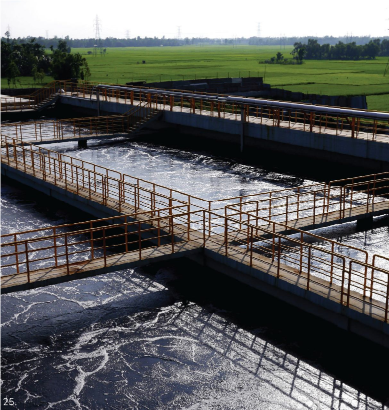
22. Inspection, 24. Shipping, 25. Effluent Treatment Plant (ETP)
