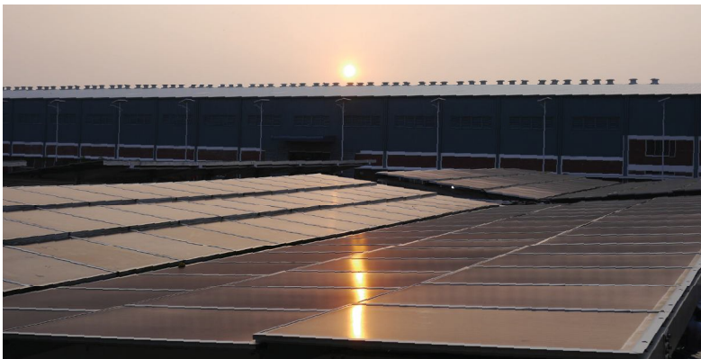
SOLAR PANELS OVERLOOKING THE PIONEER DENIM PLANT
